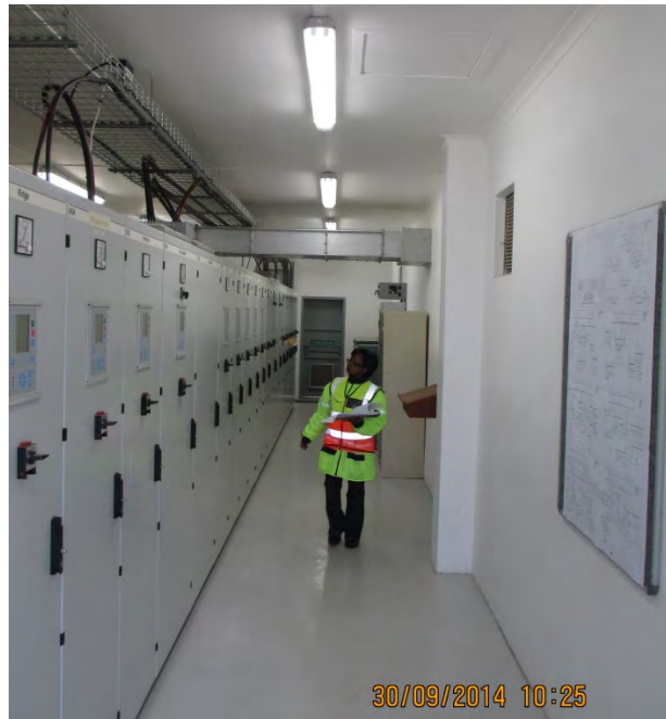
Figure 4-1 : Newly Upgraded Suidwal Substation
