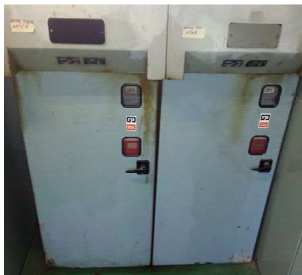
Figure 4-2 : Oil-filled Switchgear at Paradyskloof Substation
